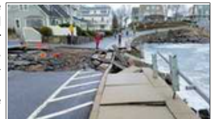
Coastal flood damage in Marblehead, Massachusetts, from the March 2-3 nor'easter. [Jim Palmer, KB1KQW, photo]
