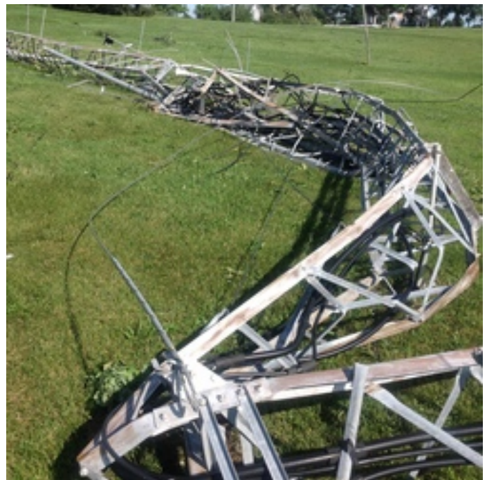
The downed 200-foot tower at W3LPL. [Courtesy of Frank Donovan, W3LPL]
