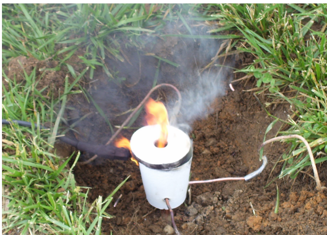
Lit Cadweld joining the grounding ring to the grounding rod at the AARC Clubhouse.
