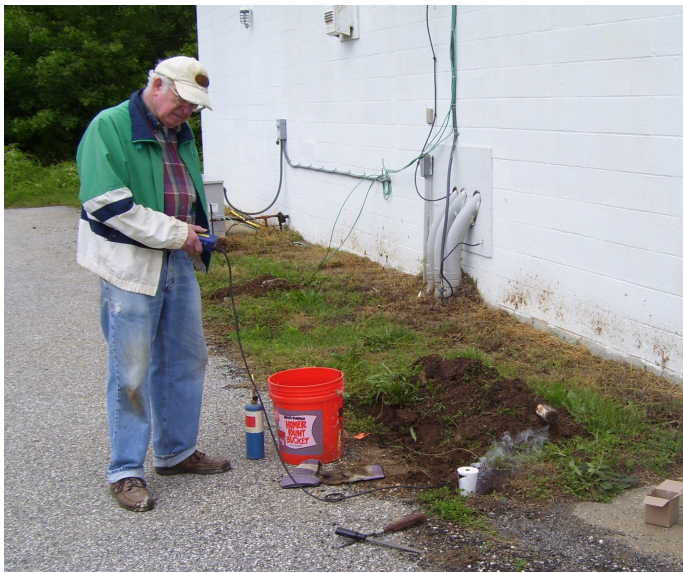
Chuck Tanner, K3ACT has activated the Cadweld to secure grounding ring to ground rod at AARC Club House.
